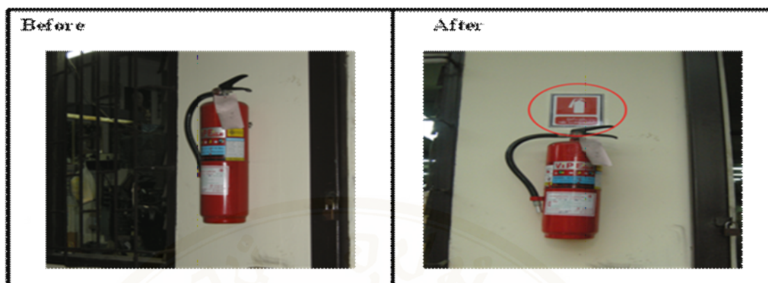
Figure 4.7 A sign showing a location of portable fire extinguisher is marked in printing factory A
