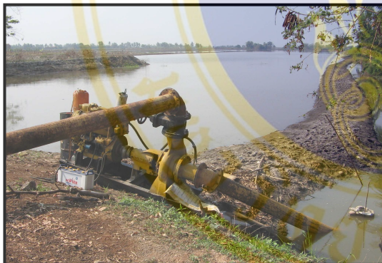
Picture 5 Water Pump as the Production Tools
